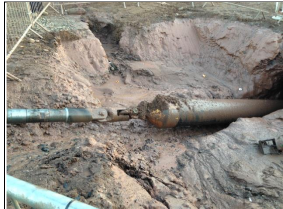
Figure 30. Drilling rod, swivel, pulling head and duct being pulled into the entry pit
