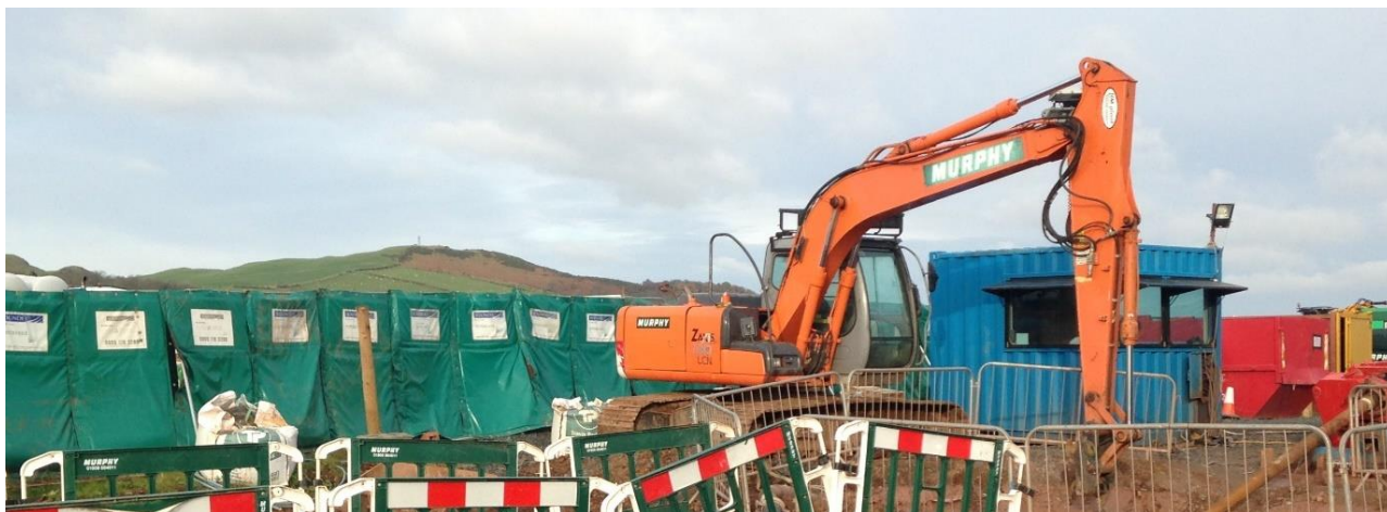
Figure 13. Noise attenuation panels on Heras Fencing on a recent UK project. The nearest neighbour was 100m from the panels. The work included allowance for 24hr working during duct installation.
