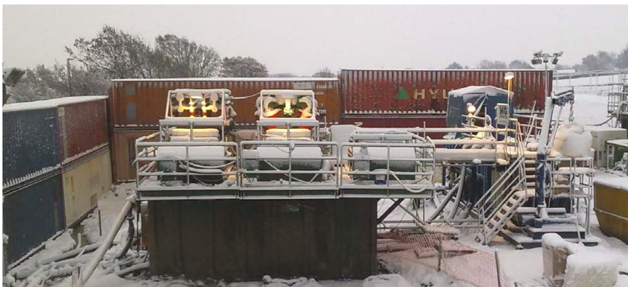
Figure 14. Stacked shipping containers used for noise attenuation panels on a UK project. There were 4 residences within 50m of the site. The work included regular evening work as well as 24hr working during pipeline installation.
