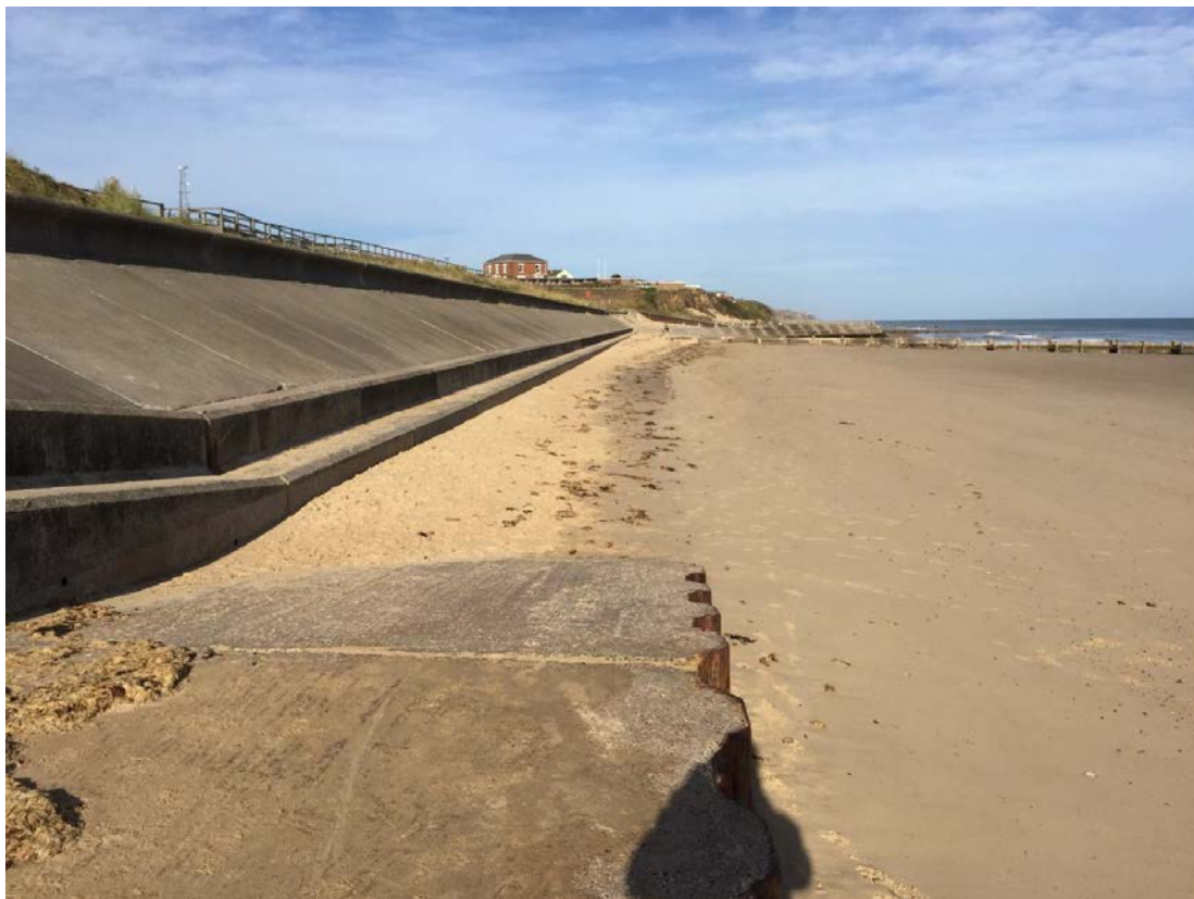
Figure 18. View W-N-W along the sea defence wall showing steel sheet piles at the toe. A timber groyne can be seen projecting into the sea in the distance.
