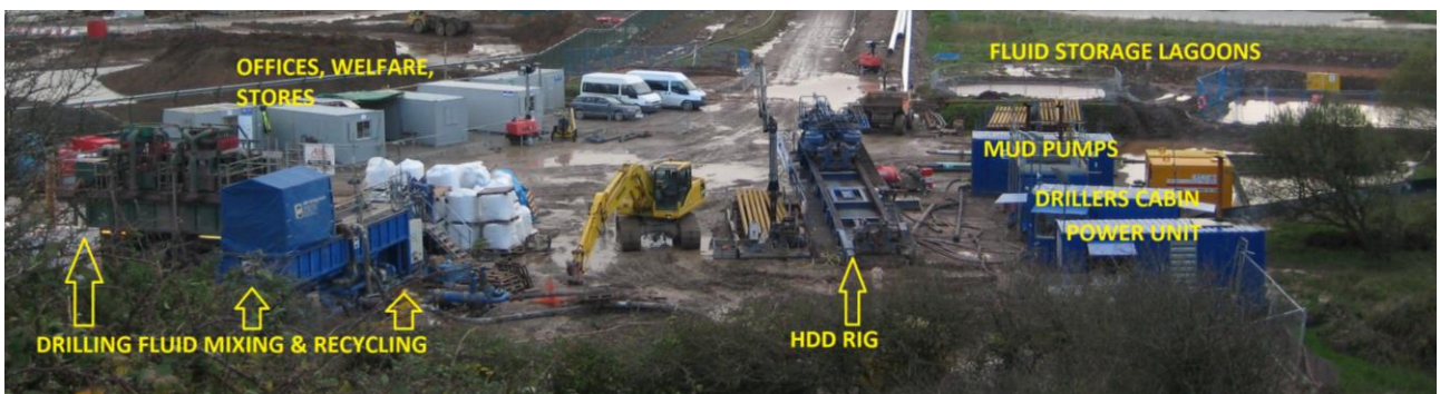
Figure 23. Example HDD site layout. Fluid storage lagoons are sometimes replaced with storage tanks.
