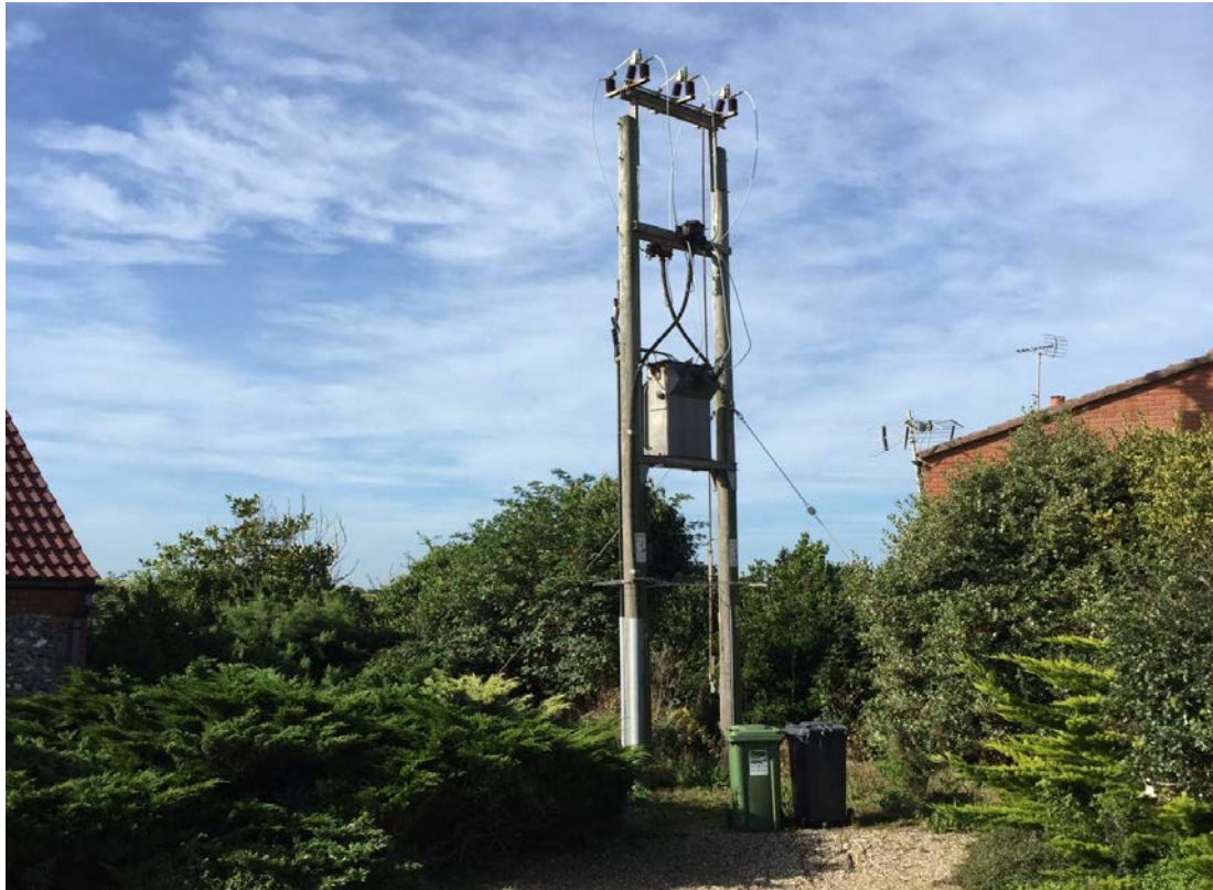
Figure 13. Transformer for underground cables located on the opposite side of the B1159 Coast Road from the site. The transformer can also be seen in Figure 10.
