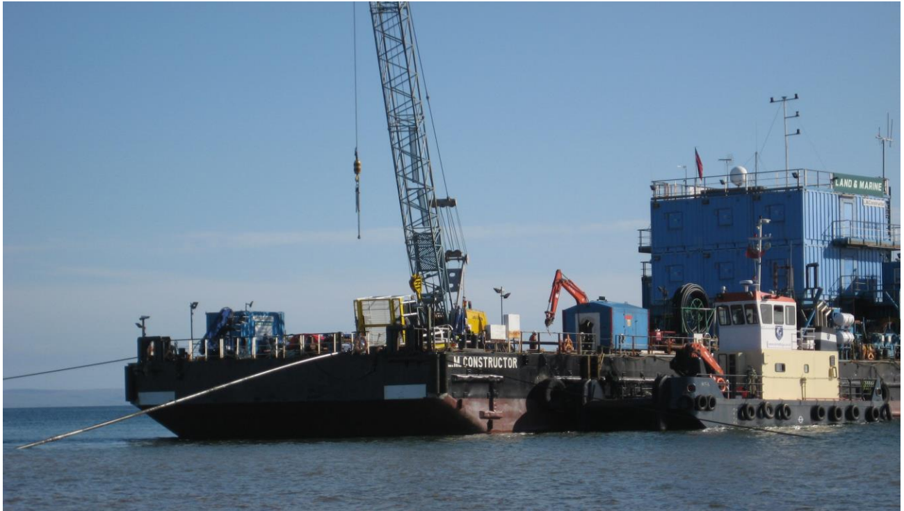
Figure 19. Pilot drilling string being pulled aboard on a UK project after an exit in 5m water.
