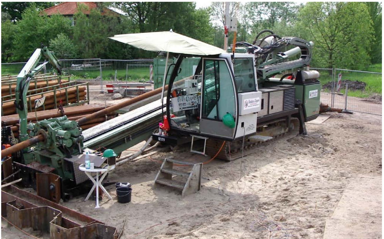
Figure 25. Example HDD rig of the midi size likely to be used for the short HDD's. A sheet piled rig anchor is visible on the left.
